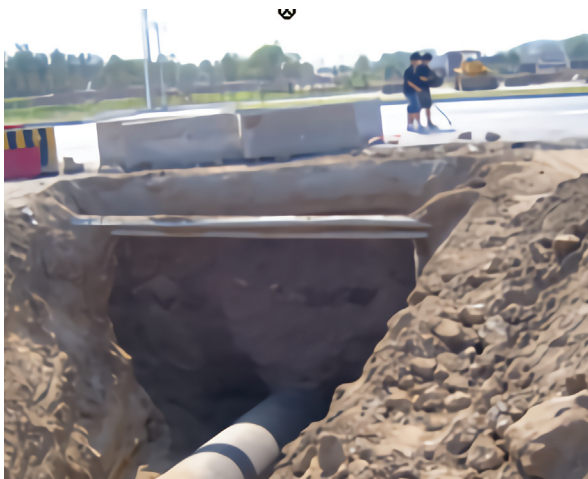
Figure 3. An exposed buried pipeline in the Changping District, Beijing.
